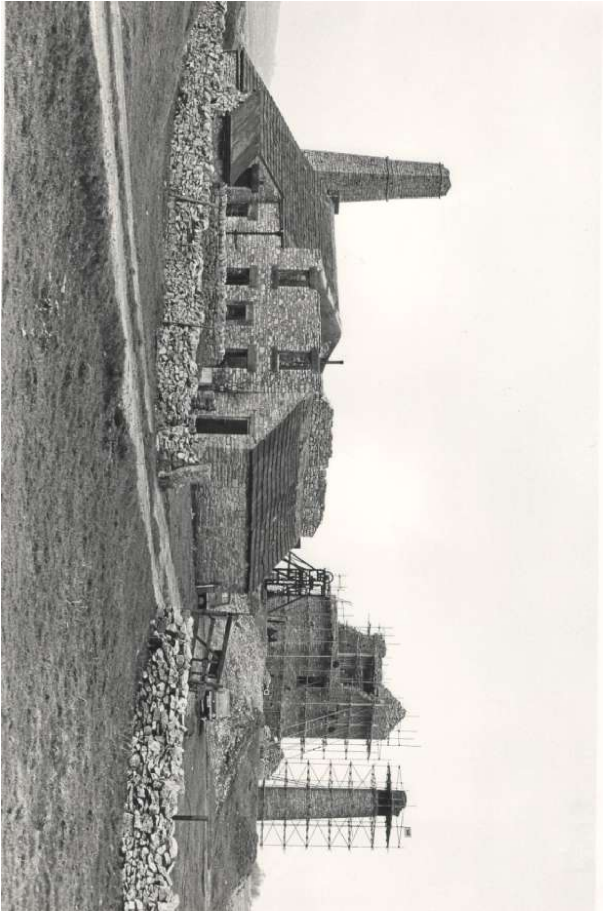
Restoration is taking place on the engine house and chimney, whilst the agent's house is still roofless, c. 1975, courtesy of H. Parker.
